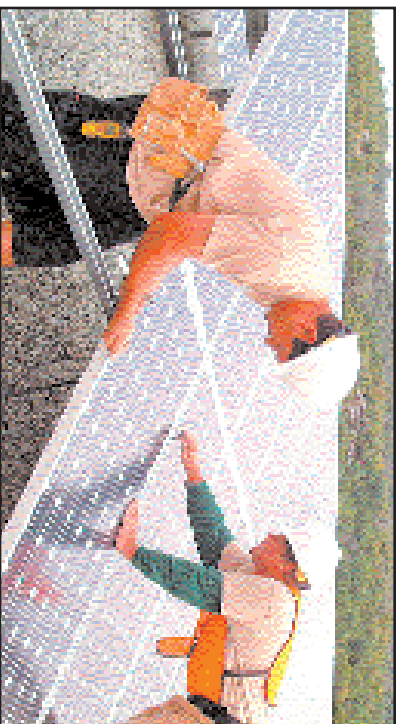
Employees of San Rafael's Sun Power & Geothermal Energy install a ground mount photovoltaic system.
